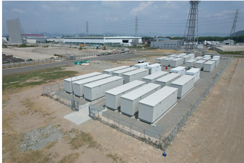
(Himeji Energy Storage Facility / Photo taken in August 2025)
